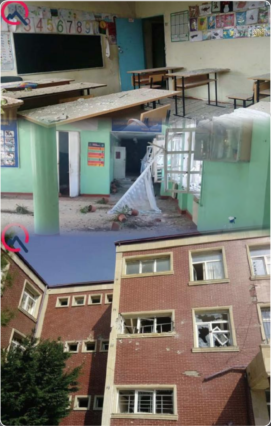
School buildings damaged in the attacks
