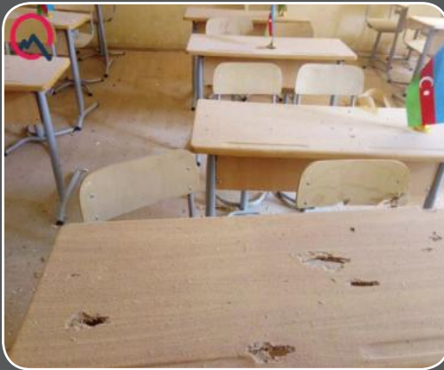
A secondary school building in Tartar damaged in the attacks
