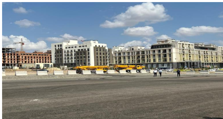
Above: Photo taken of the construction work being carried out to build new residential areas in Fuzuli city which includes hospitals and schools
